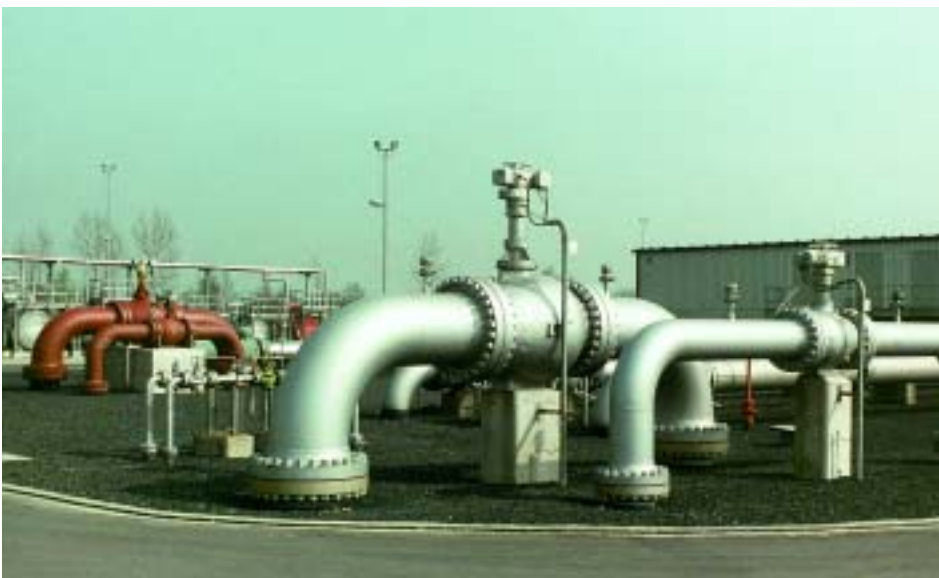
flow control valves, underground gasstorage field Germany
