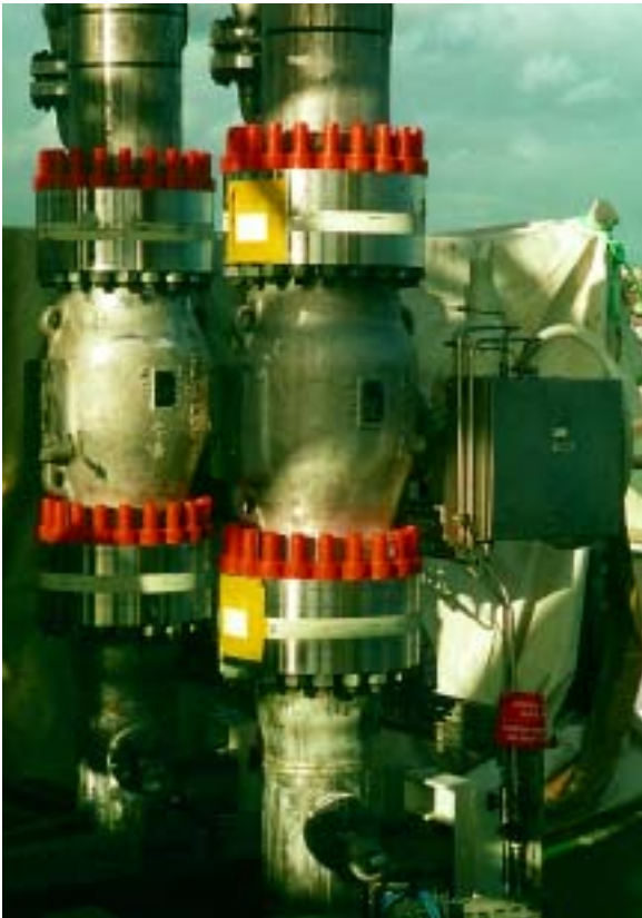
inline production chokes 10" ANSI 1500, FPSO Norway
