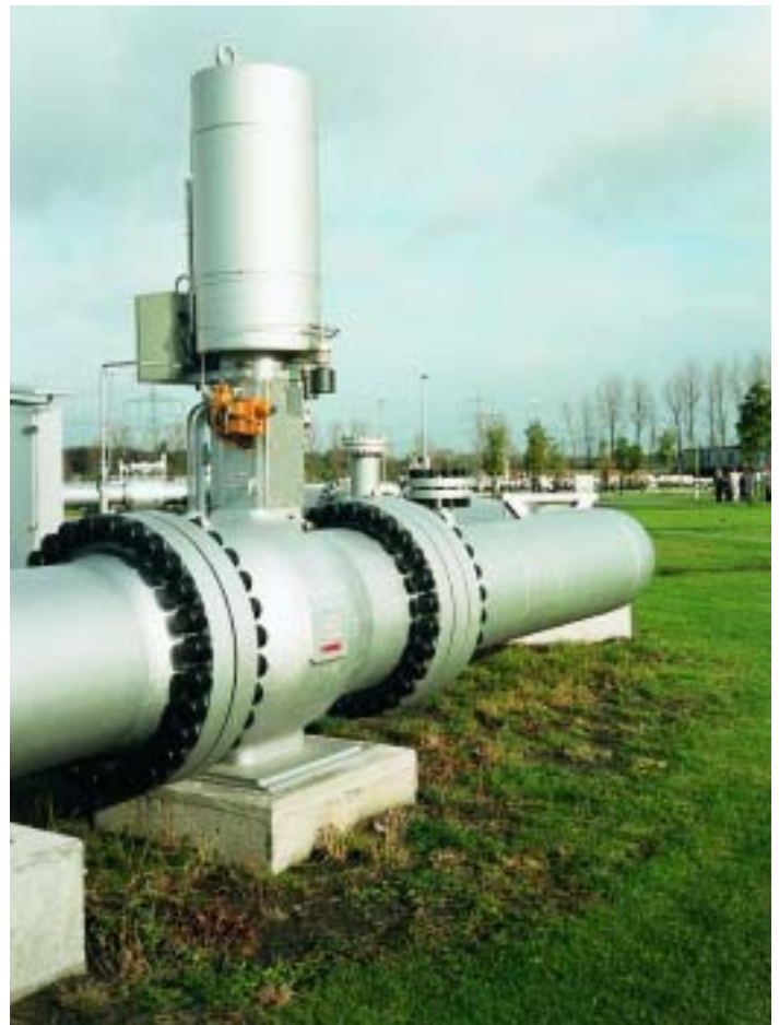
HIPPS valve 28" ANSI 600 lbs in natural gas booster station, Germany
