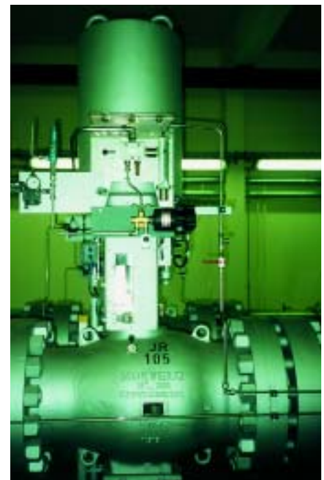
safety shut-off valve 16" ANSI 600, underground storage field Germany
