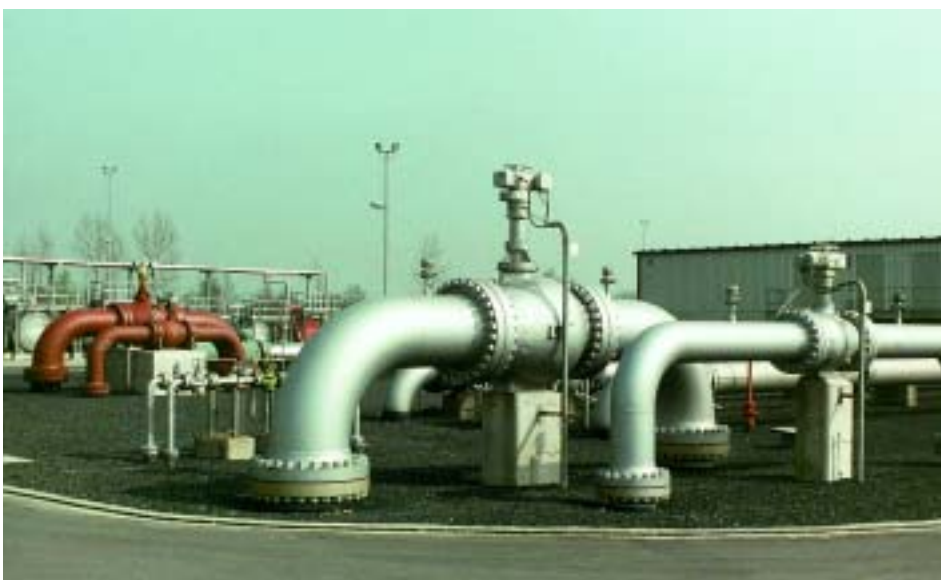
flow control valves, underground gasstorage field Germany
